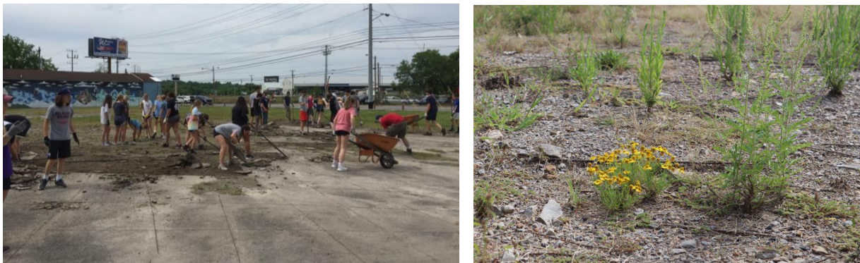
Figure 5 Depave Nashville Brown's Creek Project: Removing 18,000 sf parking lot, Native vegetation replaces parking lot (Source: https://cumberlandrivercompact.org/portfolio/browns-creek-depave-project/ )
